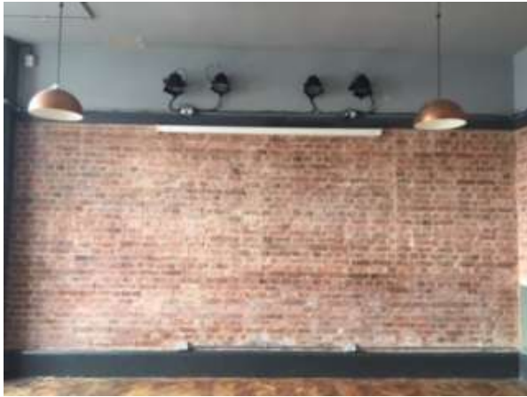
LED Pars and pull down screen on back wall
