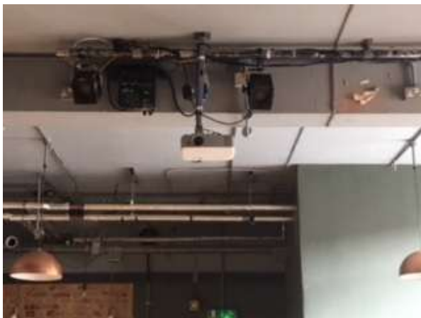
FOH bar showing Minim's, Dimmer and Projector
